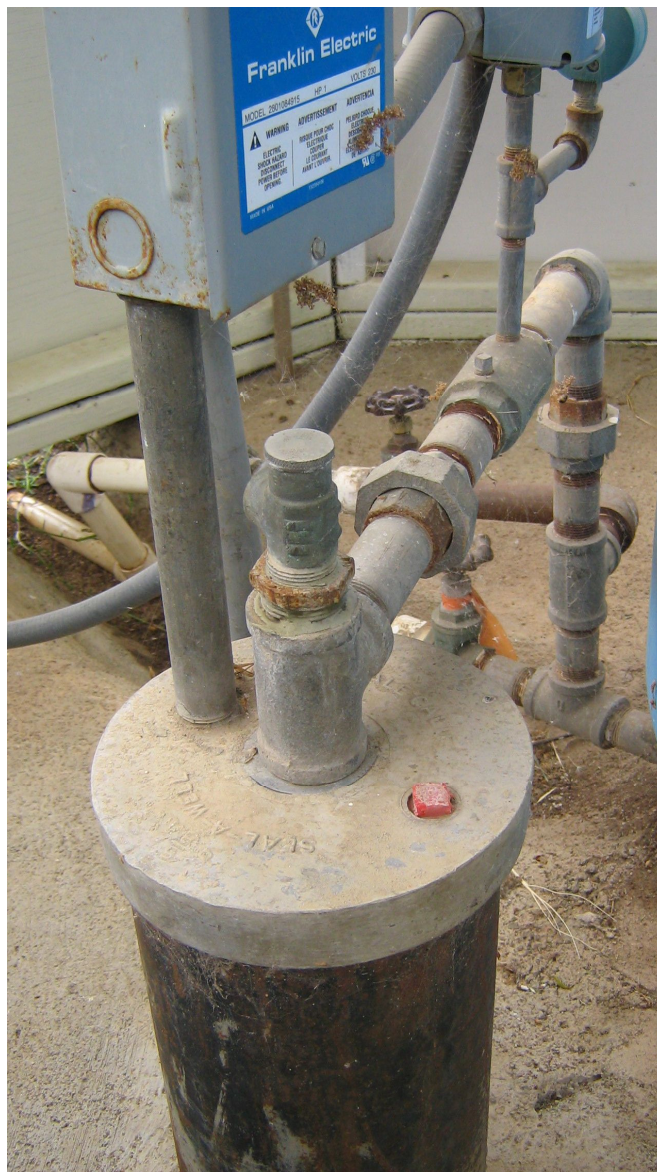
Photo: A domestic well showing the well casing, cover, and conveyance system. The well is located inside a shed with a concrete floor.
